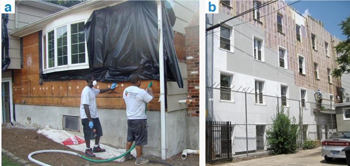
Insulation methods for existing walls Photo (a): Drill and fill for wall cavities Photo (b): Overclad insulation retrofits
